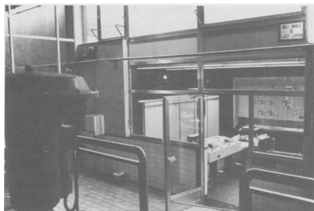
FIG. 27. General view of central control room for refinery process computer.
